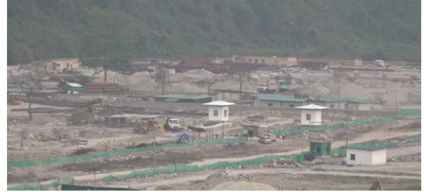
Figure 35: Norbugang Industrial Park at a glance
